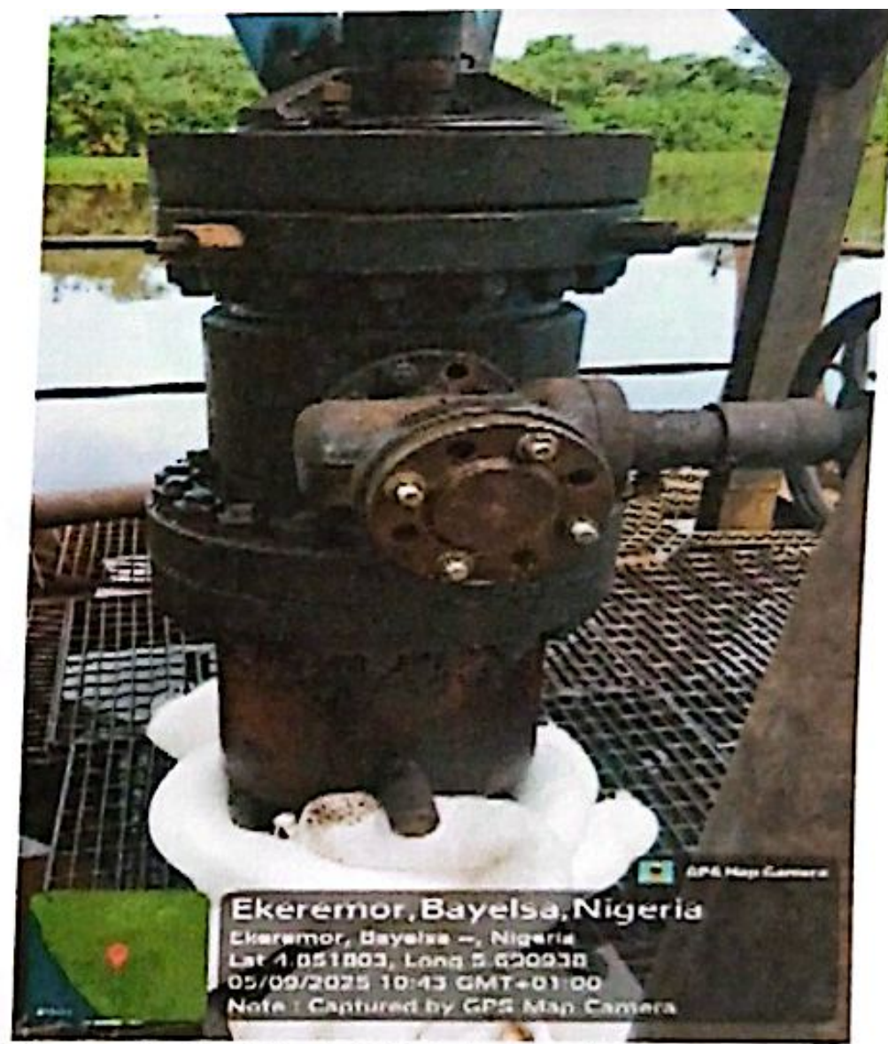
Figure 2: Incident Point during inspection
